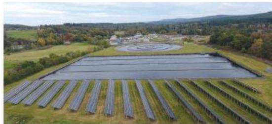
Photovoltaic solar panels at Invercarnie Water Treatment Works
